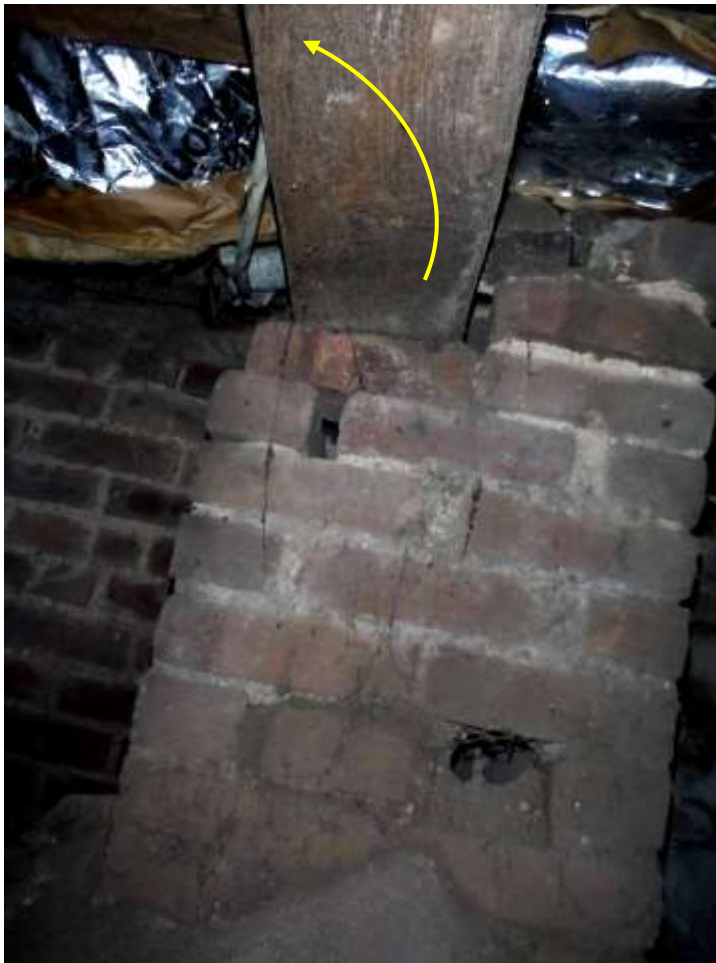
Figure 22 Damaged columns and warped framing ( joists, beams, subflooring/flooring, etc.).
