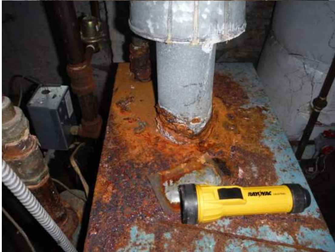
Figure 28 Boilers unsafe not tested/part removed/apart; unsafe/not functioning.
