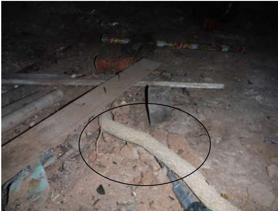
Figure 21 Tree roots, debris, nails/boards (unsafe) conditions.
