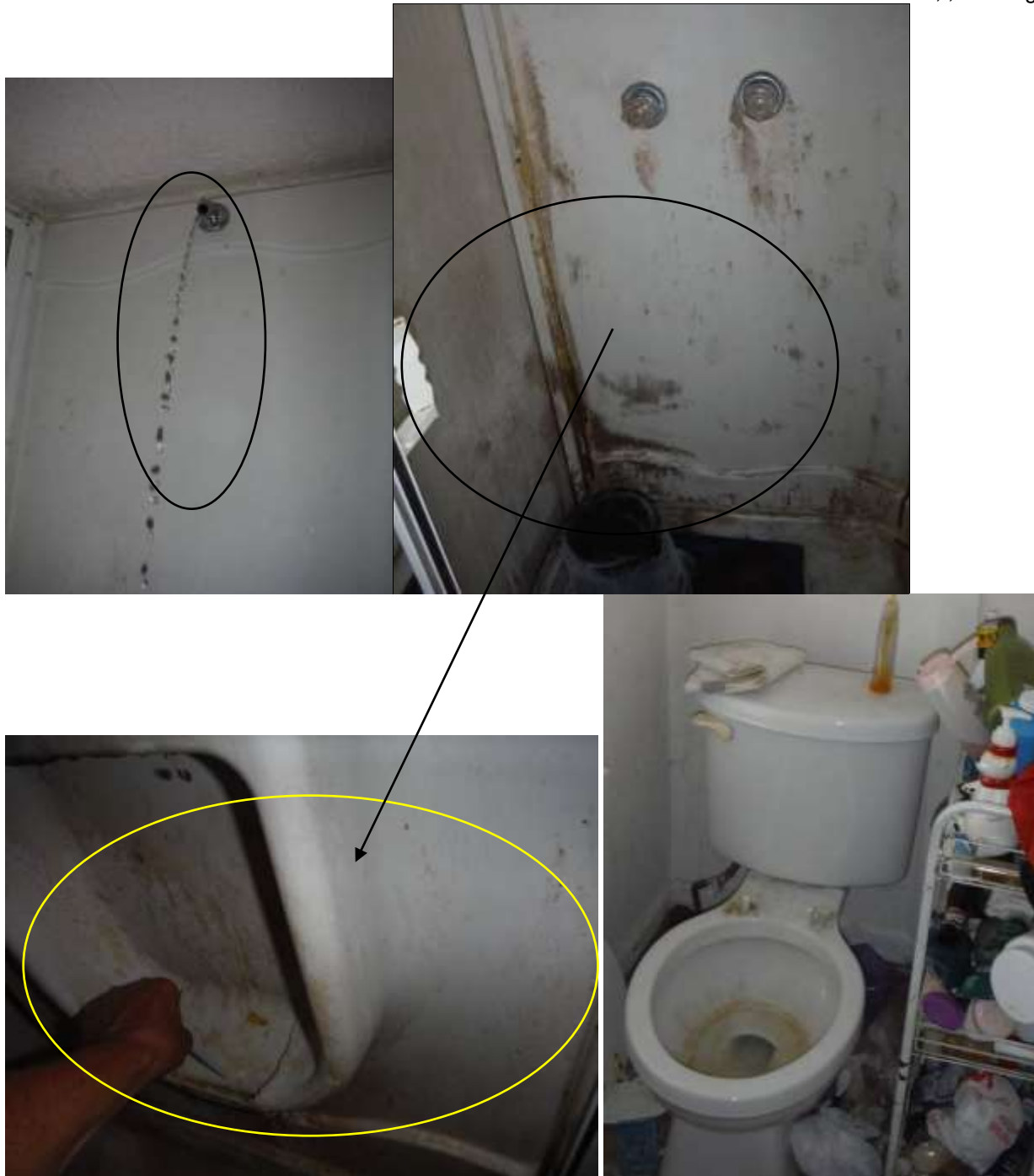
Figure 26 Unusable bathroom; need gutting, upgrades, plumbing & electrical in the home. Water damage, mold-like substances in the home. Recommend a mold contractor or environmental company evaluate all mold and asbestos and environmental substances; beyond the scope of a home inspection.
