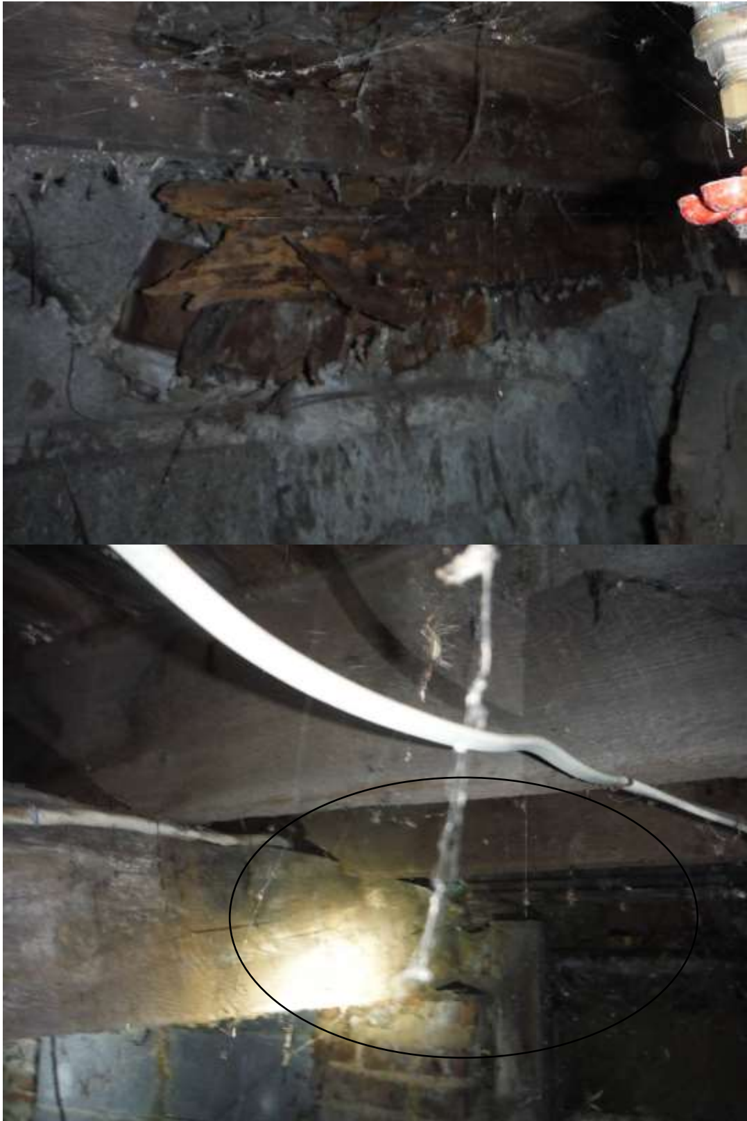
Figure 23 Example of column, girder and floor joist structure damage; extensive. Recommend a structural engineer (PE) and building contractor evaluate extent of water/mold/fire damage in the home. Sub flooring, joists and beams or framing breaking up when touched or probed. There is indication of water & fire damage in the home. Flooring in all floors were warped and spongy; concealed or inaccessible on upper levels.
