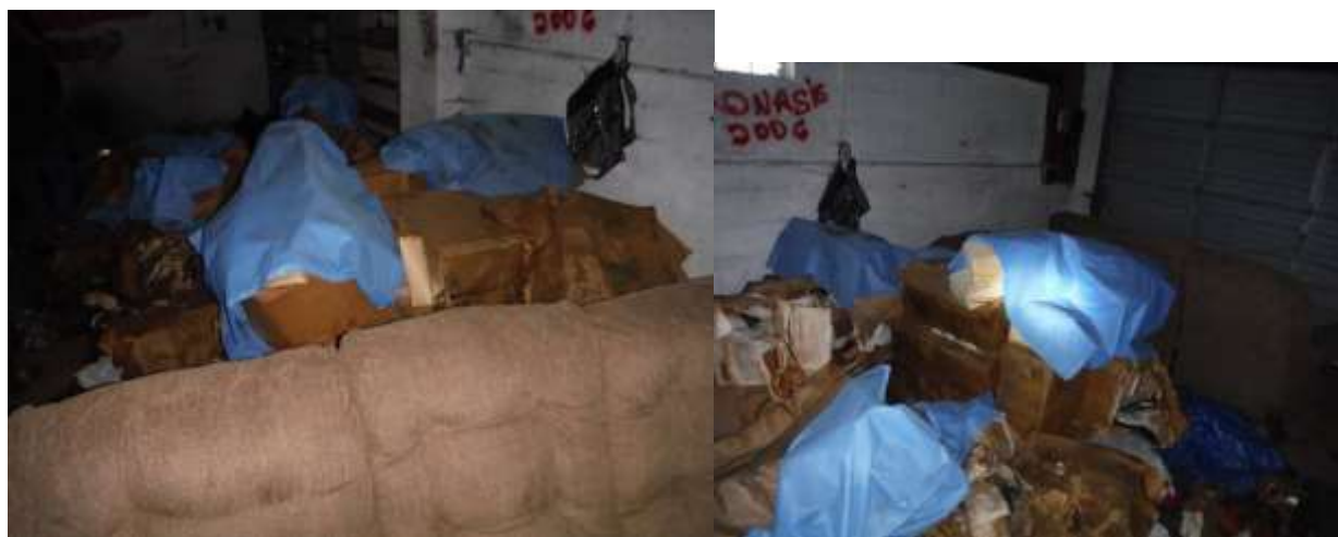
Figure 8 Wet/moldy rotted storage in garage.
