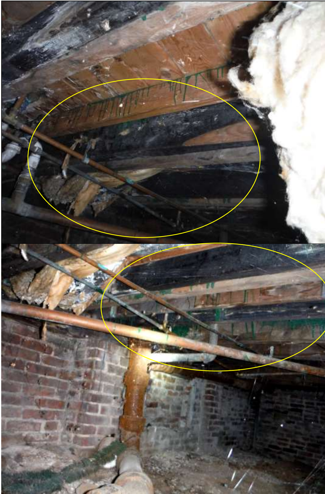
Figure 20 Examples of charred/fire damaged wood in rear crawl space. All structure must be evaluated by a structural engineer (PE) and advise on all repairs. Flooring was warped and spongy in the home. Obtain all history for fire & water damage before closing.
