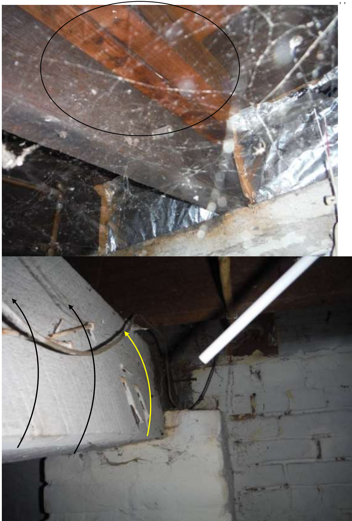
Figure 18 Twisted main beam/girder in basement. Floor joists and beam were sagging, flooring/subflooring spongy/deflection or movement when walked upon; structural defects/deficiencies observed in the home.
