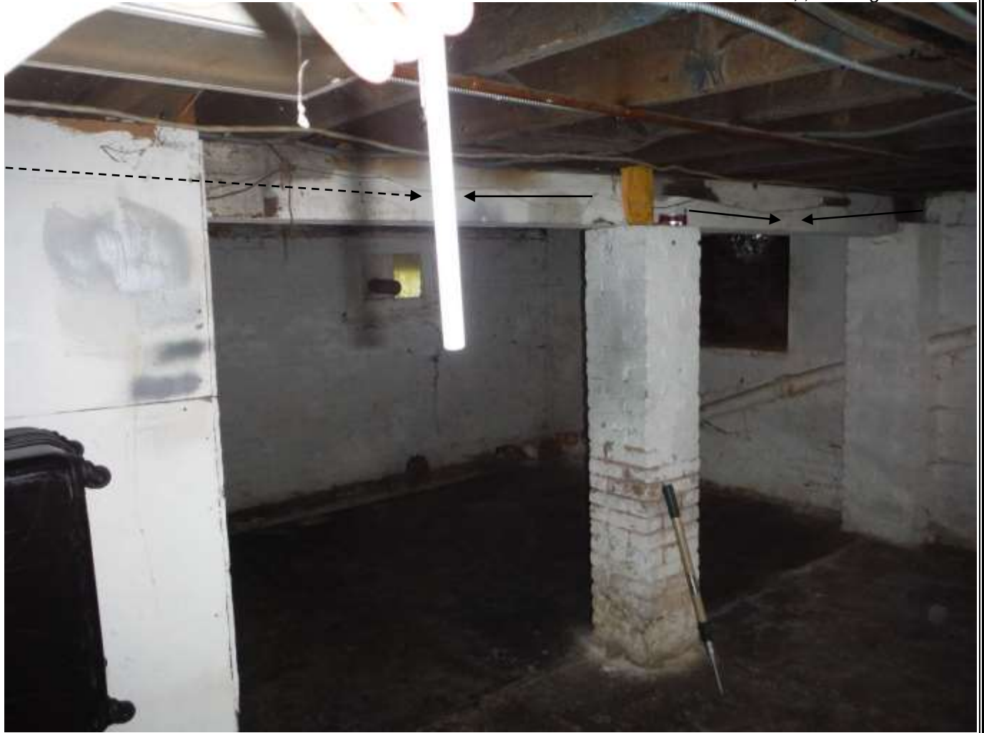
Figure 17 Sagging twisted beam/girder. The girder and floor joists were sagging, sloped spongy flooring/damaged throughout the home.
