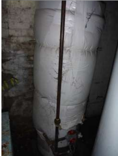
Figure 27 There was no hot water in the home at time of inspection. Water heaters and boilers were in poor/unsafe condition. Recommend a licensed plumber and boiler contractor evaluate all mechanicals for replacement. These must be replaced; dangerous condition.
