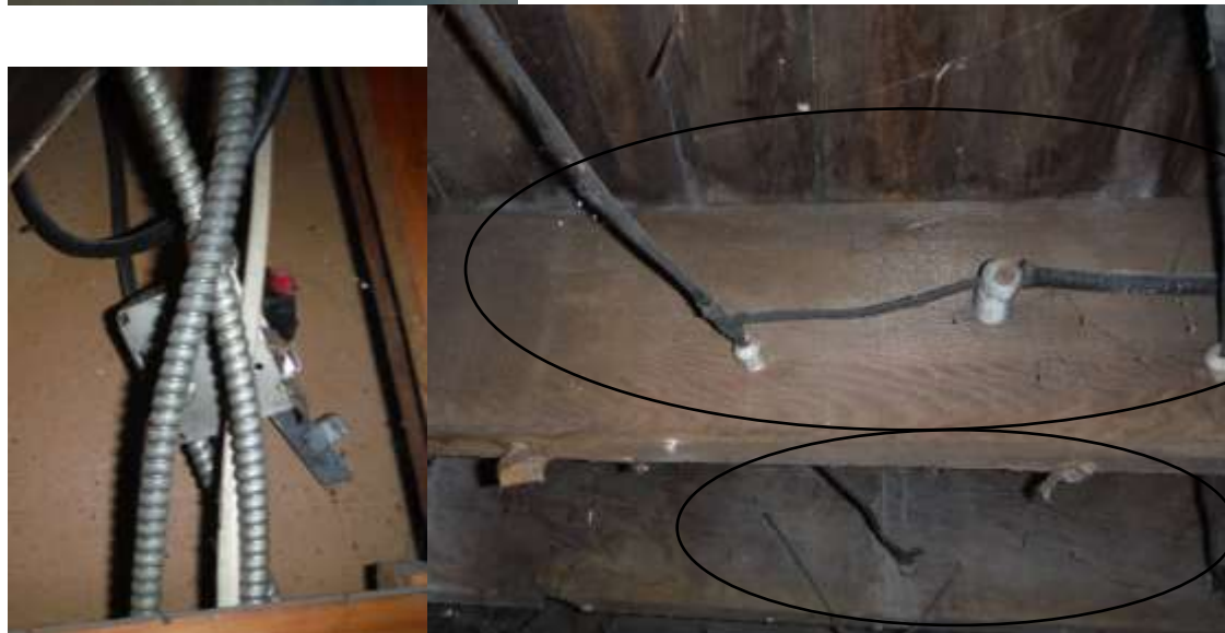
Figure 30 Examples of electrical concerns. See garage section comments.
