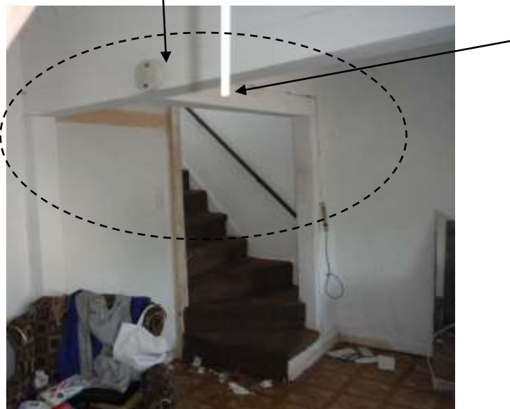
Figure 12 Sagging, sloped flooring, indication of removed walls/altered structure, etc.
