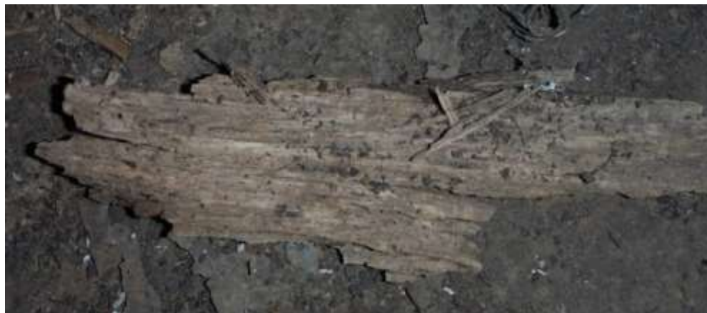
Figure 7 Example of water and wood destroying insect damage in garage.
