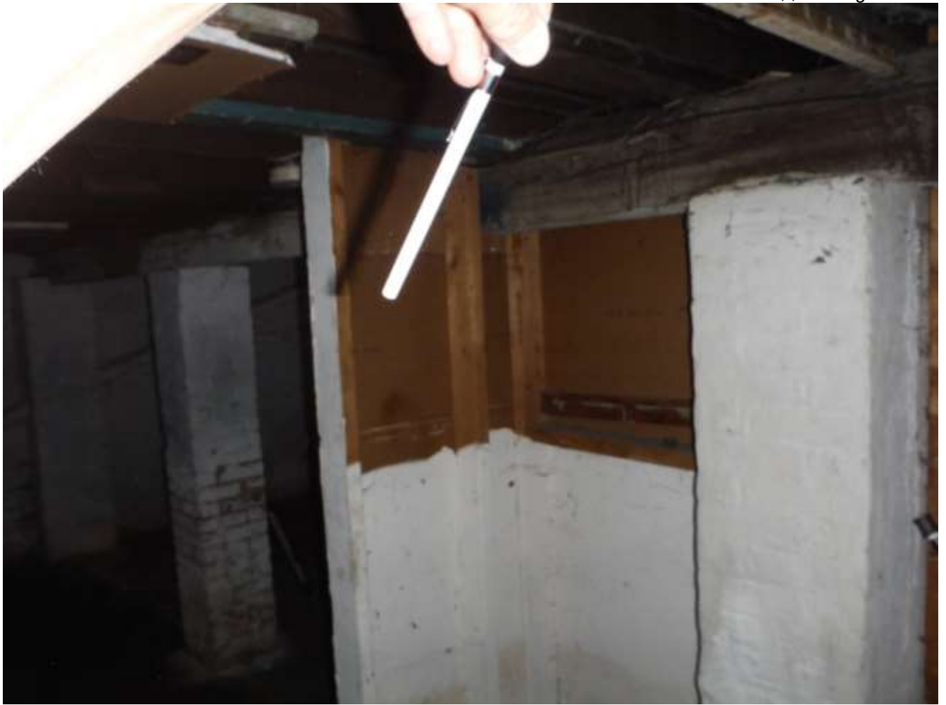
Figure 15 Main beam/girder sagging between brick columns. Center columns > 8ft. apart (should be less than). Deterioration and water damaged columns.
