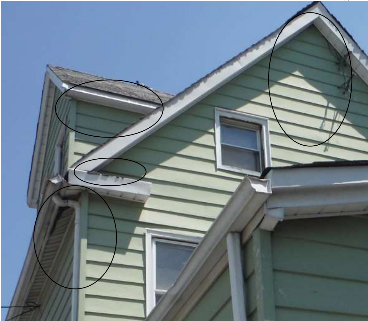
Figure 1 Roofs in poor condition; leaking into interior, water damage, etc. Have all water, mold-like and structure damage determined by building contractor and roofer.
