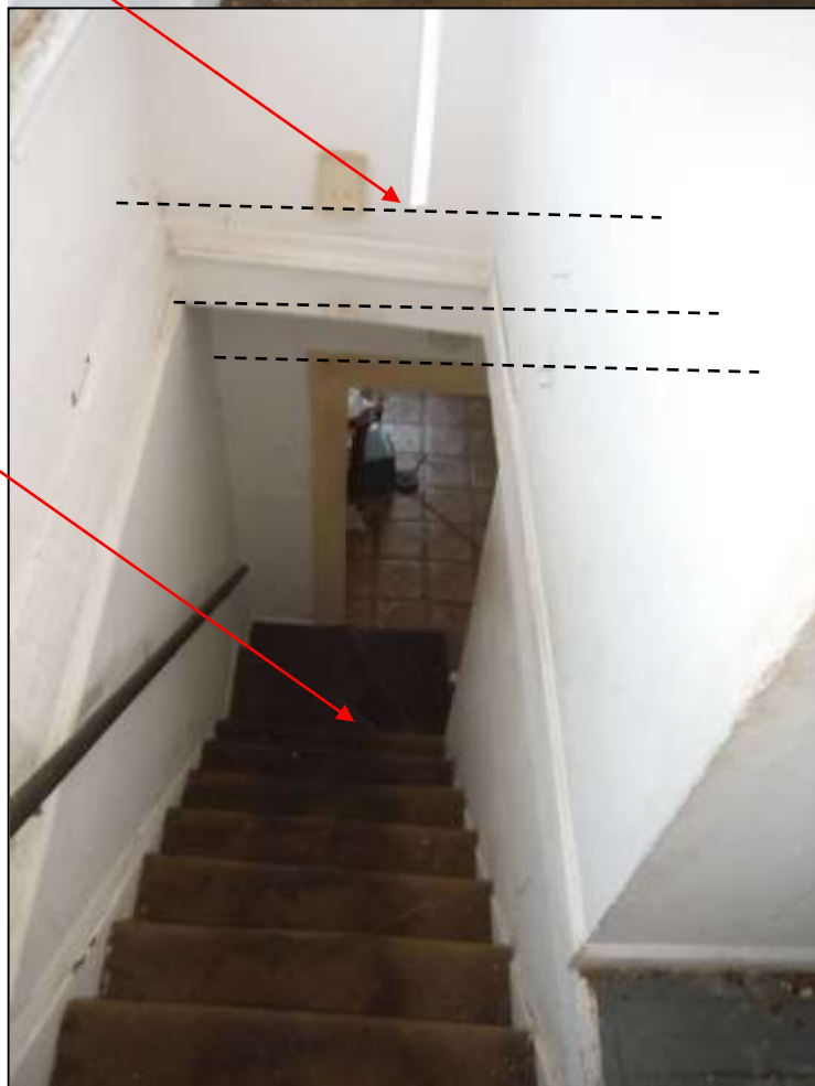
Figure 13 Sloped staircases, canted walls/doorways, etc. in the home; structural concerns. Recommend a structural engineer (PE) evaluate all structure in the home. Recommend obtaining all history for structural modifications, removed walls, fire damage, etc. before closing and contractual limitations. Stairwell to 3rd floor had trip/fall hazard; open first step off landing.
