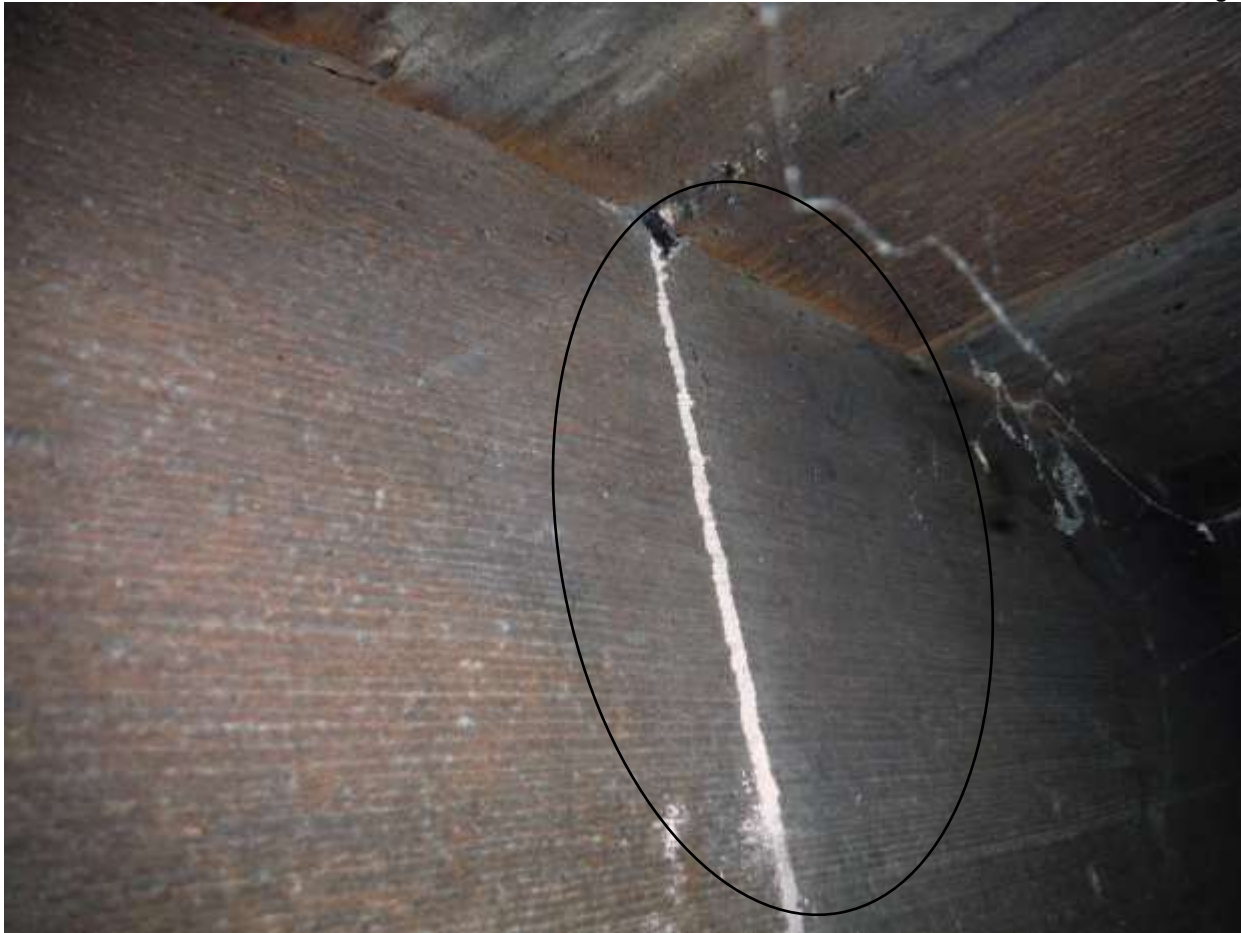
Figure 19 Example of termite shelter tubes on joists or framing. See crawl space section comments.
