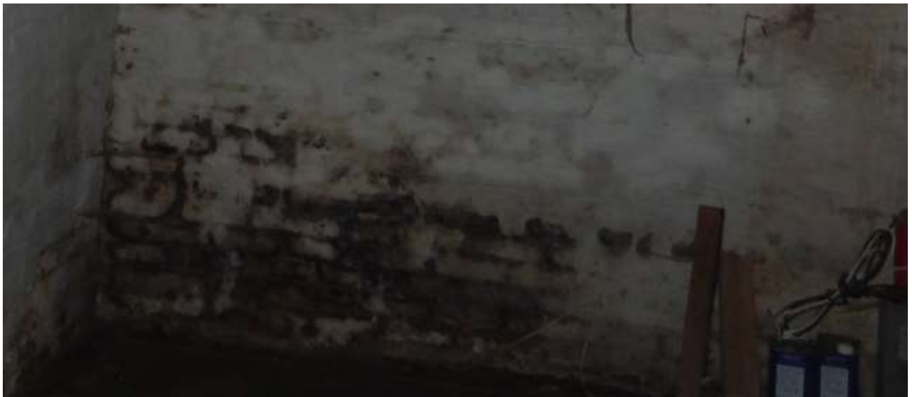
Figure 16 Mold-like staining; have evaluated by mold/environmental contractor.
