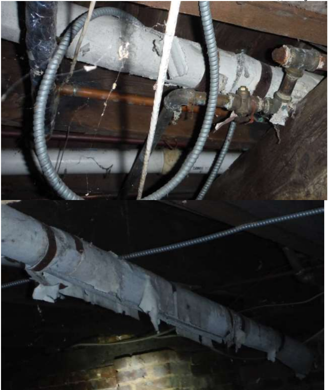
Figure 29 Example of white asbestos-like insulation on heating pipes in the home.
