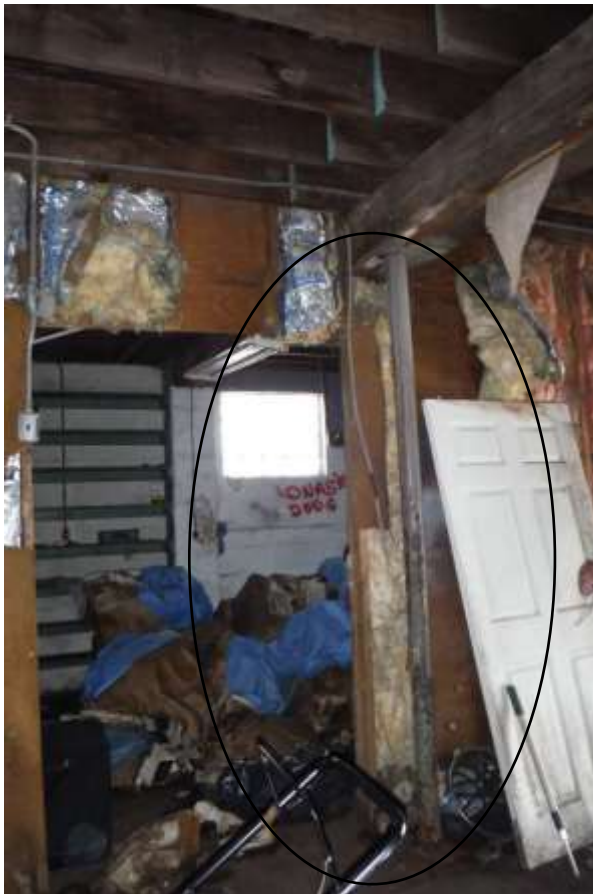
Figure 10 Rusted lally column, structural modifications, leaking roof/leaks/damaged roof structure, etc. Recommend a structural engineer (PE) and building contractor evaluate/advise on all repairs.
