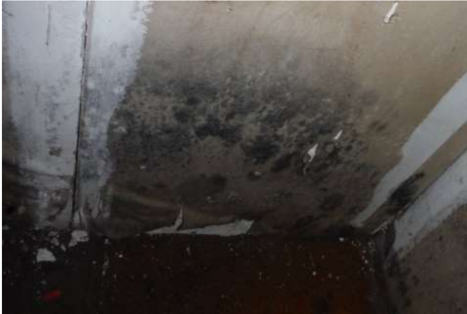
Figure 9 Example of mold-like conditions.
