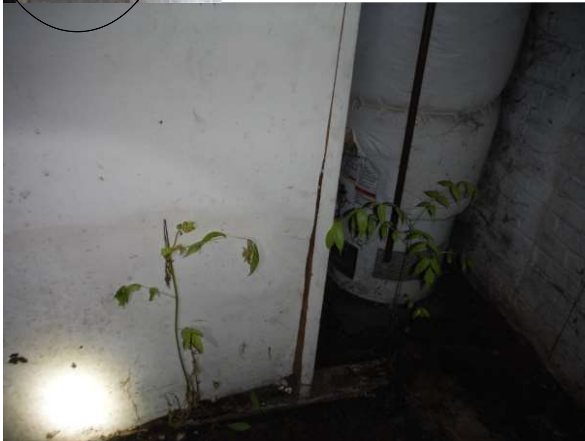
Figure 14 Wet basement & plants growing in floor around basement.
