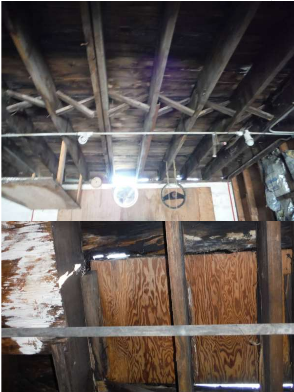
Figure 5 Holes/daylight in garage roof everywhere; extensive damage to roof /structure; have a roofer & building contractor evaluate & advise on tear off & mitigation/rehab.
