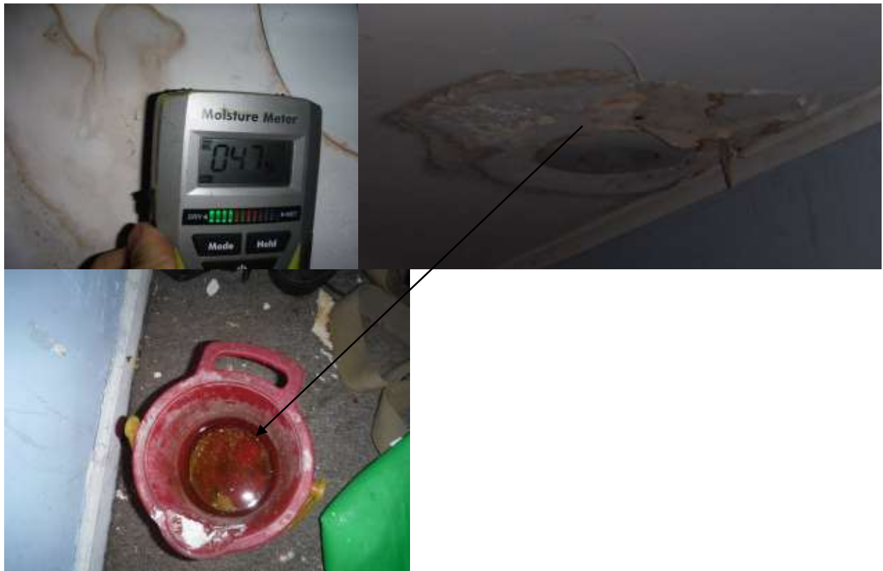
Figure 3 Water leaking through a ceiling light; dangerous.
